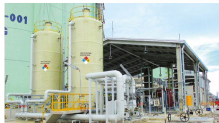
System over view/providing whole system including engineering
