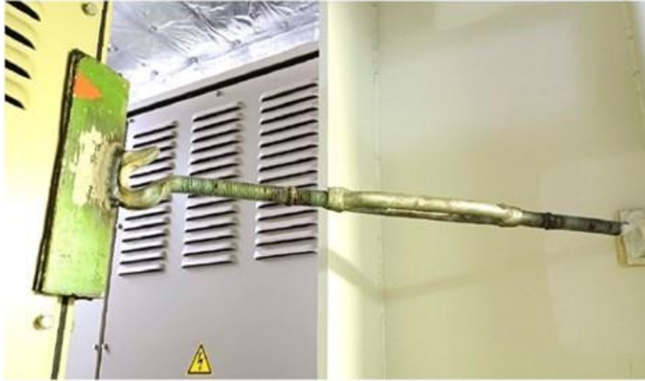
Cargo chain turnbuckle, welded to angle iron, and wedged between the number 1 step-down transformer (left) and a steel beam (right).
