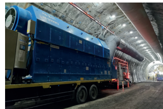
Large dust collector (3,000 m 3 /min)
