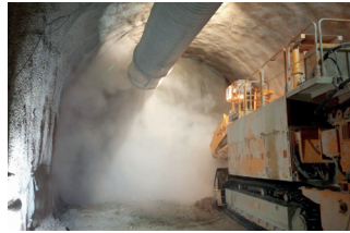
Dust collector to process dust from blasting in tunnel
