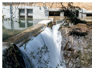
Water intake of Sukawagawa hydro power plant
