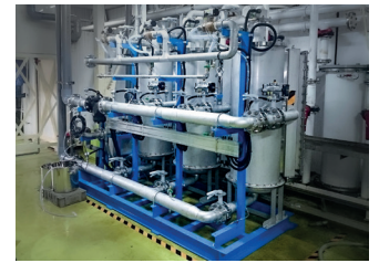
ECO Clean LFP for PFAS treatment
