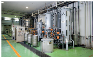
Resin processing plant
