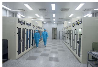
Plant site: filling & packaging
