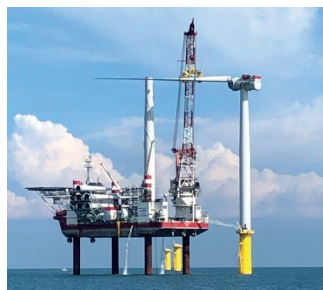
Offshore wind farm
