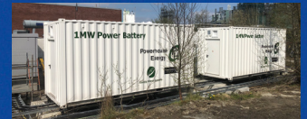
Battery storage system of Exergy Power Systems
