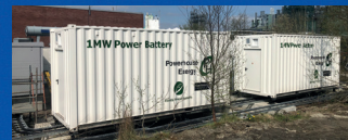
Battery storage system of Exergy Power Systems
