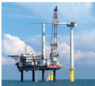
Offshore wind farm
