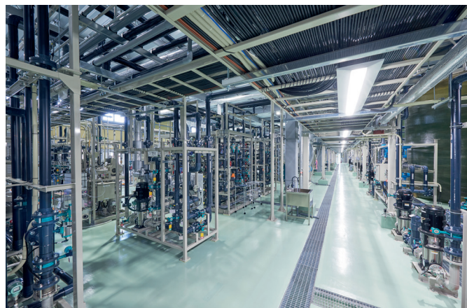
Next generation UPW system at R&D center
