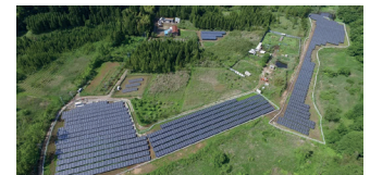
Solar photovoltaic plant in Chiba prefecture
