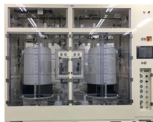
Chemical dilution and delivery system
