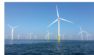
Offshore wind farm
